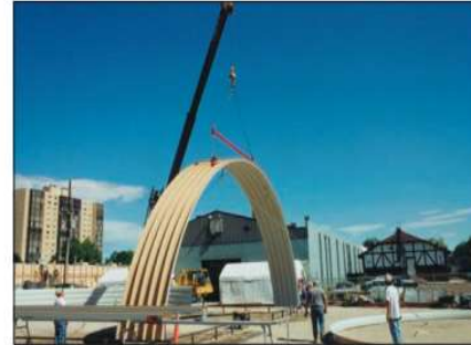
Five curved arches are seamed together on the ground, and set in place on the foundation steel.
