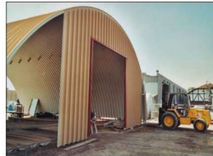
Door and window frames are installed as the end walls are being erected.
