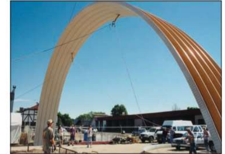
First group of arches are tied off to hanger brackets, plumbed and squared, and welded in place.
