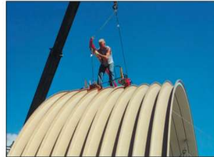
Next set of arches are nested over the first set, seamed together and welded to the foundation steel.
